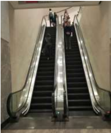
Figure 3.33 Acceptable standard escalators with Glazed edges
