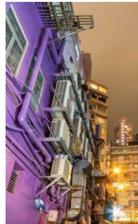
Figure 4.11 External air conditioning should not be exposed
